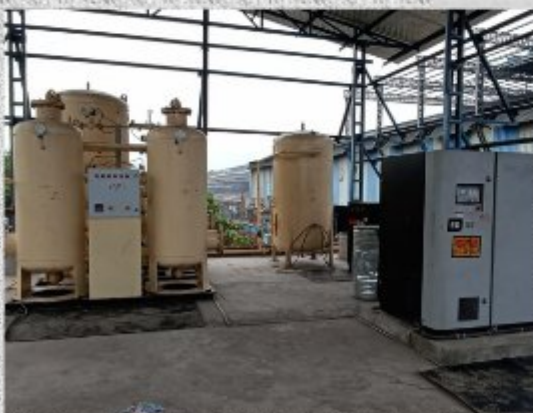
Oxygen Gas Plant
